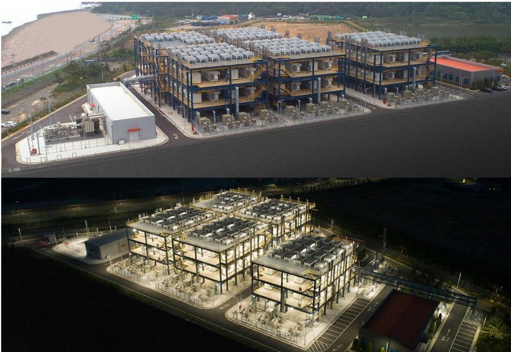
Figure 2: 50 MW PureCell® Model 400 Hydrogen fuel cell plant
